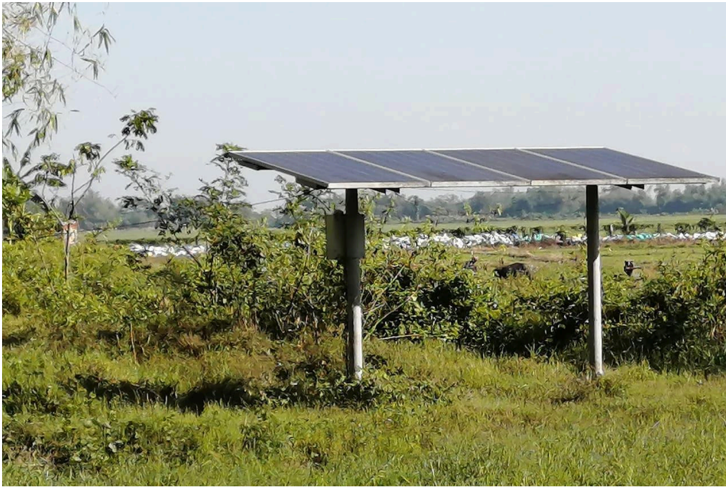
6.5.4j. Solar power-driven submersible pumps installed on dug wells and shallow wells in various locations inside the campus
