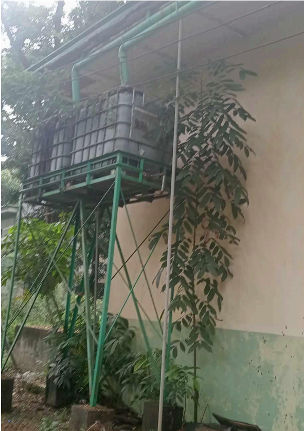
Figure 6.3.4a. Water harvesting tanks installed in one of the buildings inside TAU campus
