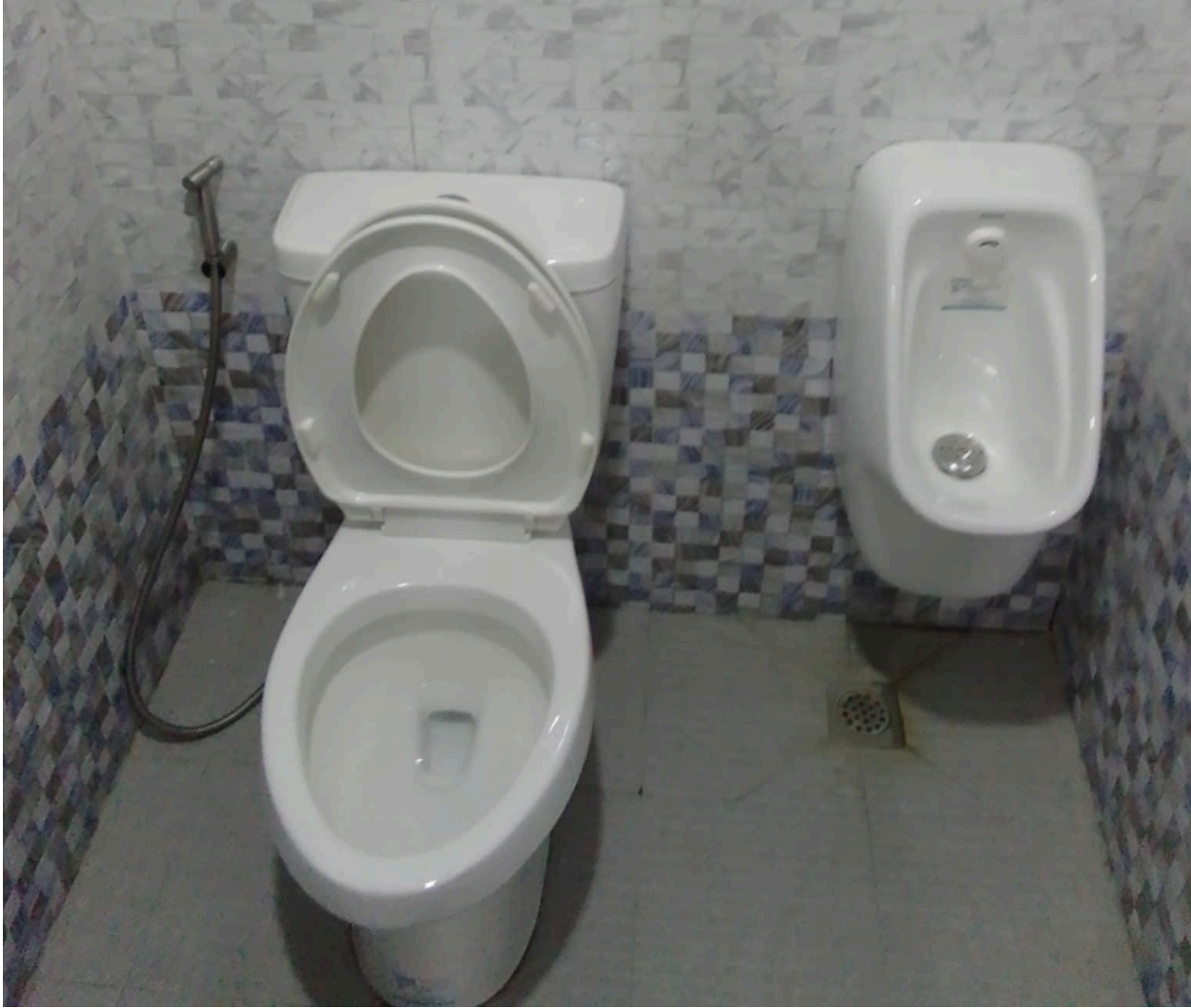
Figure 6.3.4a. Sensor-operated urinals and water-saver water closets
