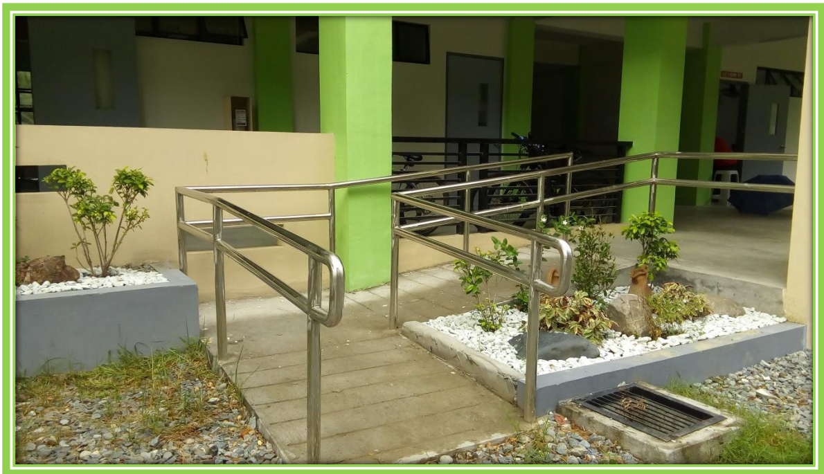
PWD Ramp at the College of Engineering and Technology (CET) Annex 2 Bldg.
