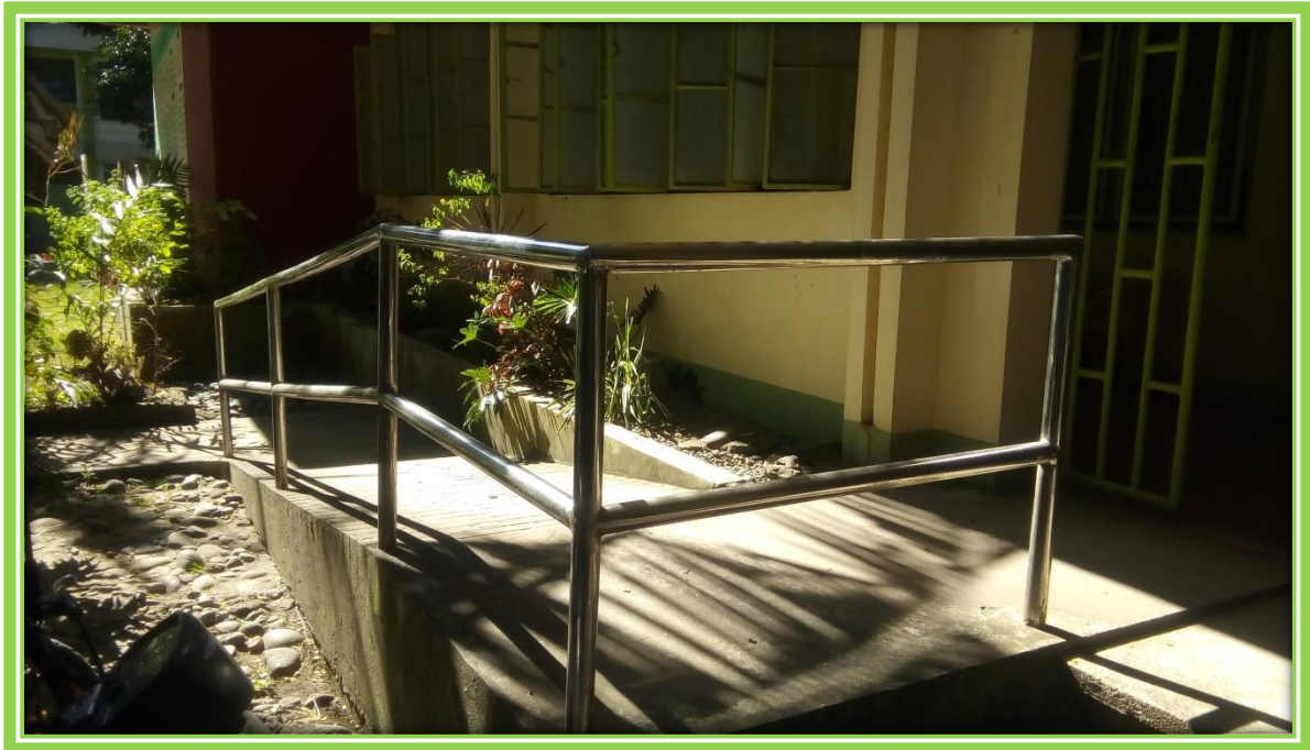
PWD Ramp at the College of Engineering and Technology (CET) Annex 1 Bldg.
